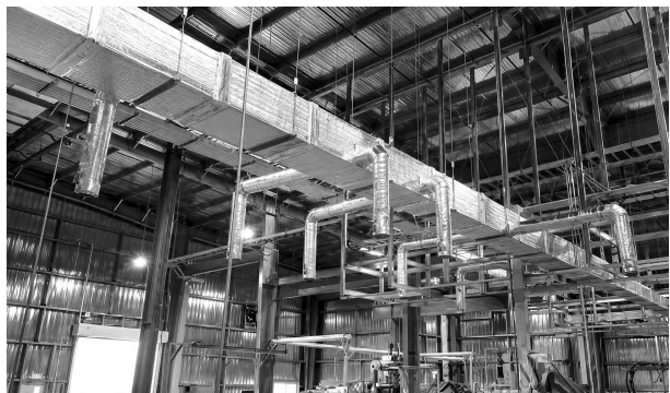
Figure 2: Ventilation system installed in the factory
